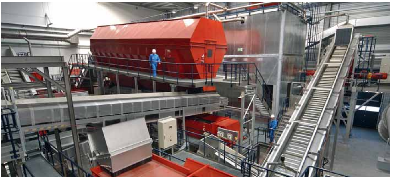
Inside the Mechanical-Physical Stabilisation Plant Reinickendorf
