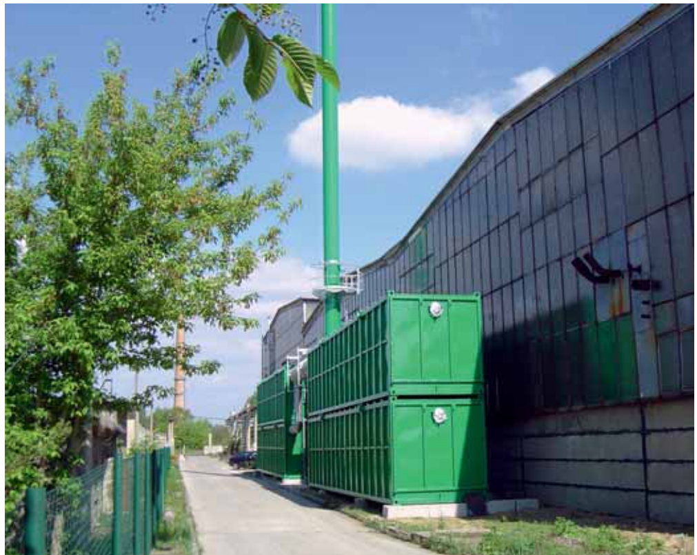
Bio-filter plant of the Mechanical Treatment Plant Köpenick
