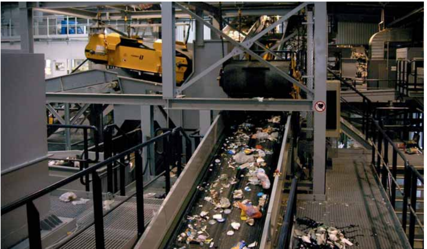
Sorting plant for lightweight packaging in Hellersdorf
