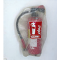
Hayatuna: Fire extinguisher
